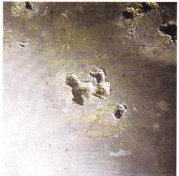
Fig. 2: Surface damage to tanks caused by micro-organisms
